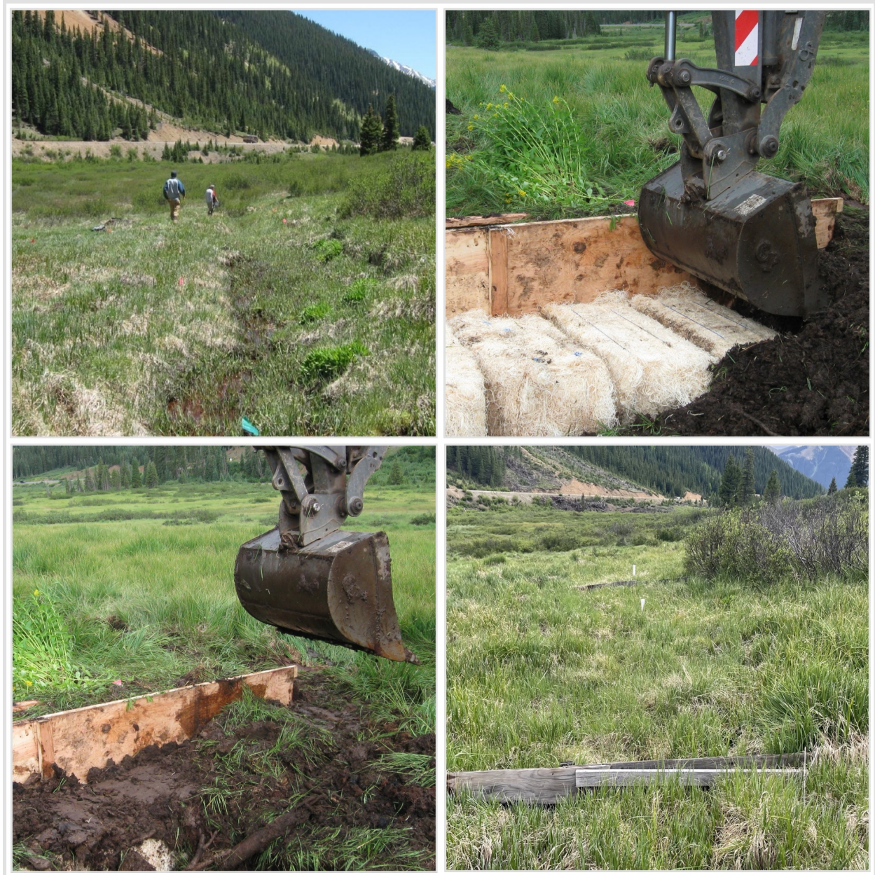
Figure 20. Using fiber bales for ditch infilling. Ditch before restoration (top left), during restoration (top right and bottom left), and five years after restoration (bottom right).
