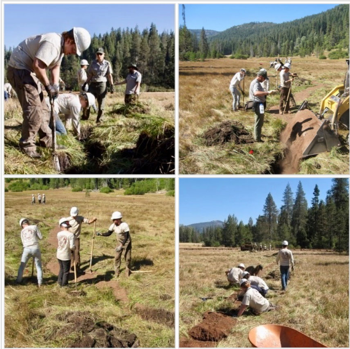
Figure 21. A 200 m long ditch in Drakesbad Meadow, a fen in Lassen Volcanic National Park, California was completely filled with sediment in 2012. The ditch was first cleaned and grubbed to make sure no undercut banks or vegetated areas were present (top left). Then the ditch was filled with sandy loam sediment (top right). The sediment was tamped to remove all voids and create a suitable planting surface (bottom left). Then plugs of vegetation removed from the grubbing stage were added back in rows across the fill material.
