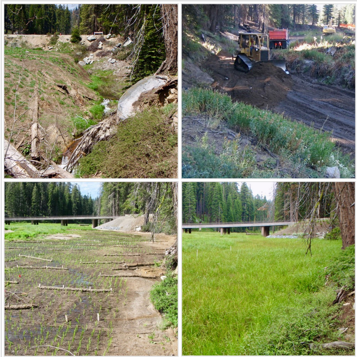
Figure 34. Gully (top left) in Sequoia National Park that was filled (top right), planted and covered with geotextiles (bottom left) and fully restored a few years later (bottom right). The road was replaced with a bridge in addition to filling the gully (top left vs. bottom photos).
