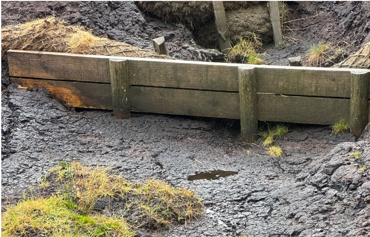
Figure 31. Example of poorly designed impervious ditch dam showing where water eroded under the dam.
