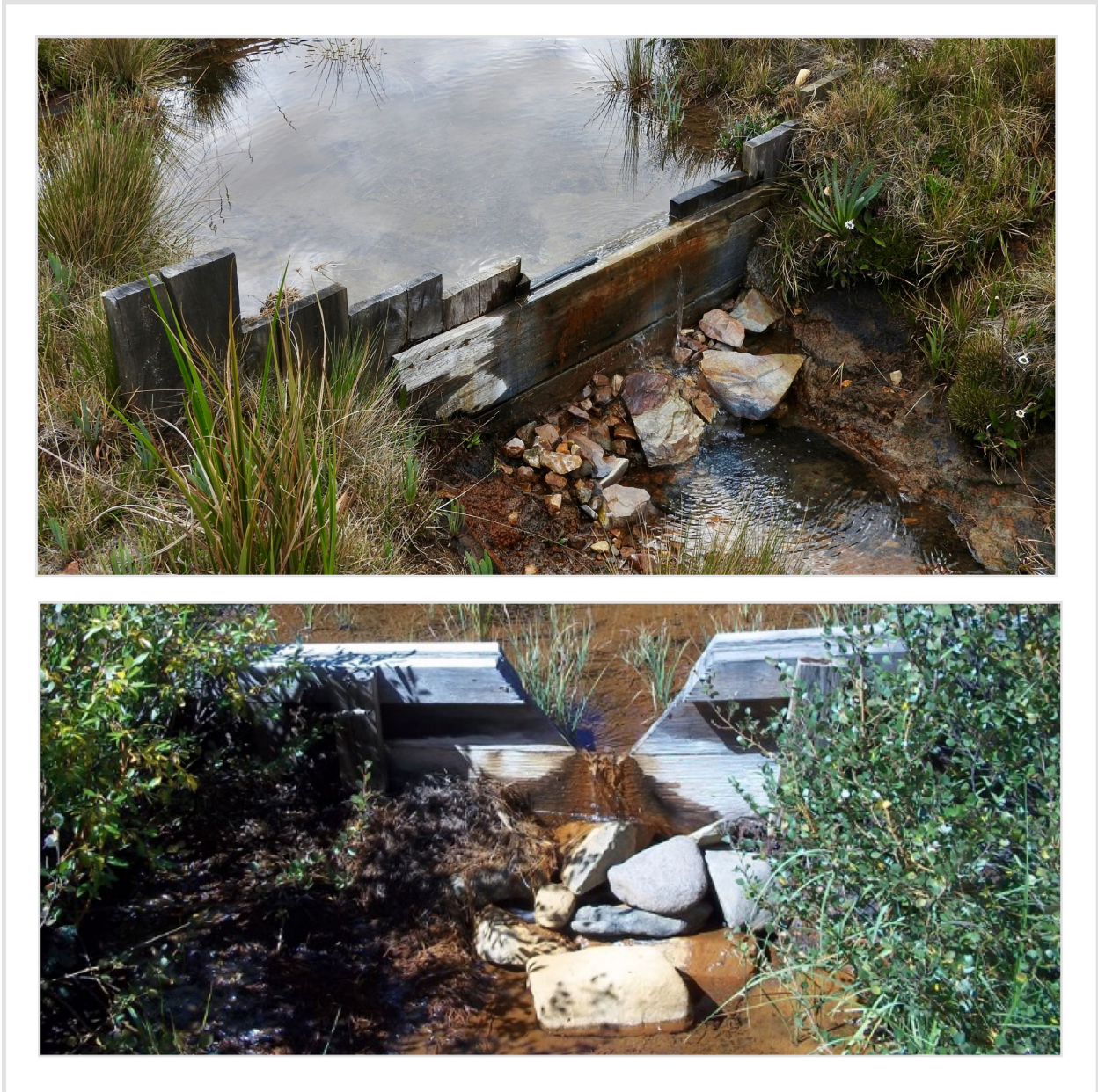
Figure 29. Two examples of wood permeable ditch dams for use in high flow ditches. Vertical wood planks (top) and horizontal wood planks (bottom).
