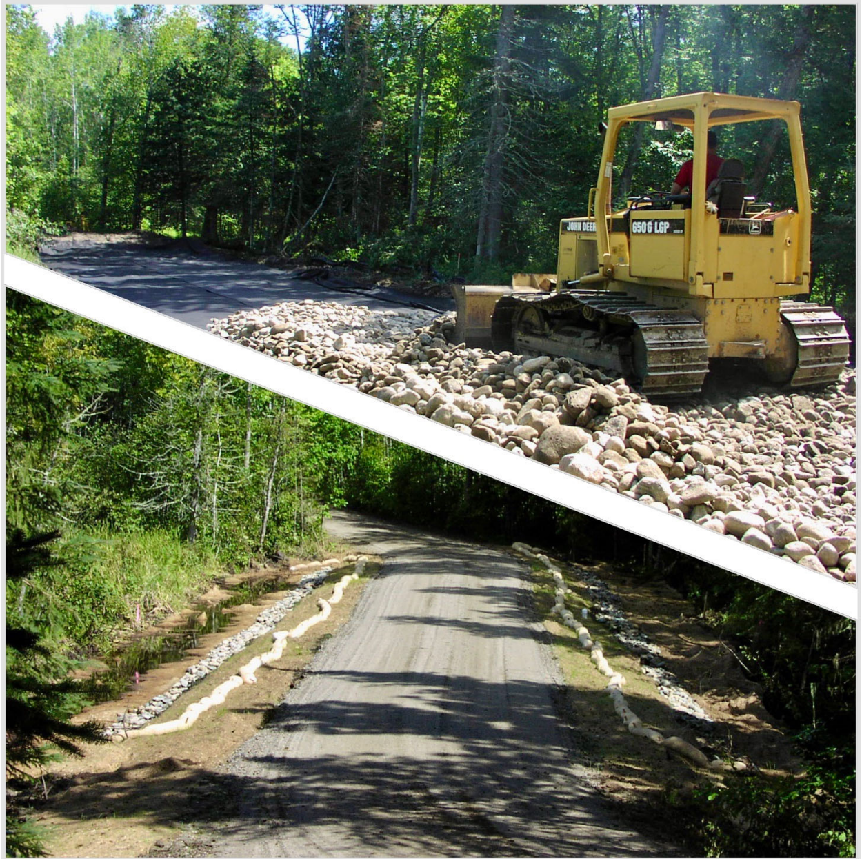
Figure 36. Construction of a permeable roadbed (top) with the finish road shown (bottom).
