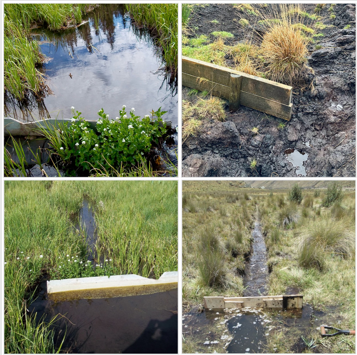
Figure 32. Example of poorly designed impervious ditch dams allowing water to flow around the dams.
