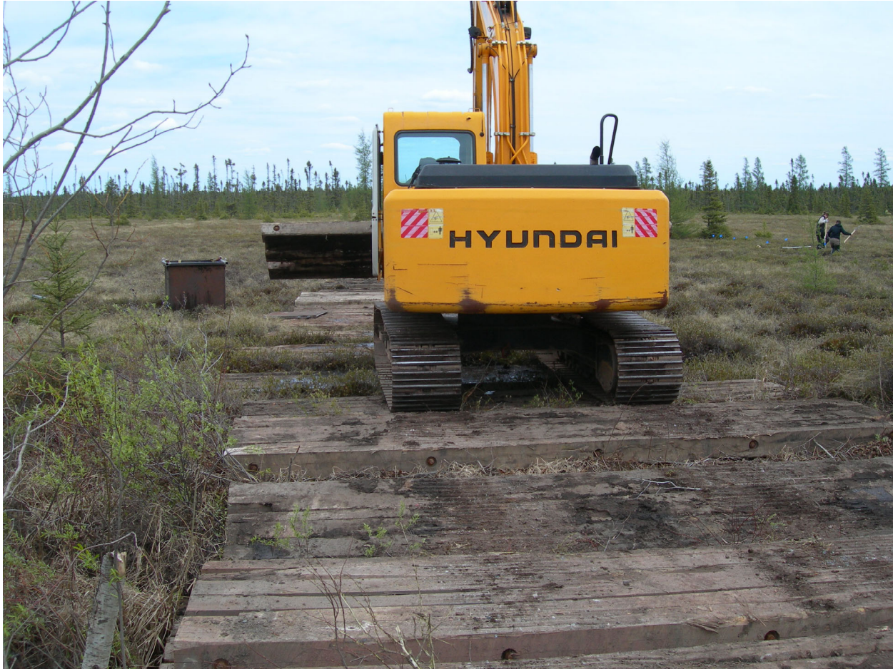
Figure 48. The use of mats can be important for driving on soft organic soil, especially where the peat is soft or equipment is not specialized for wetland work.
