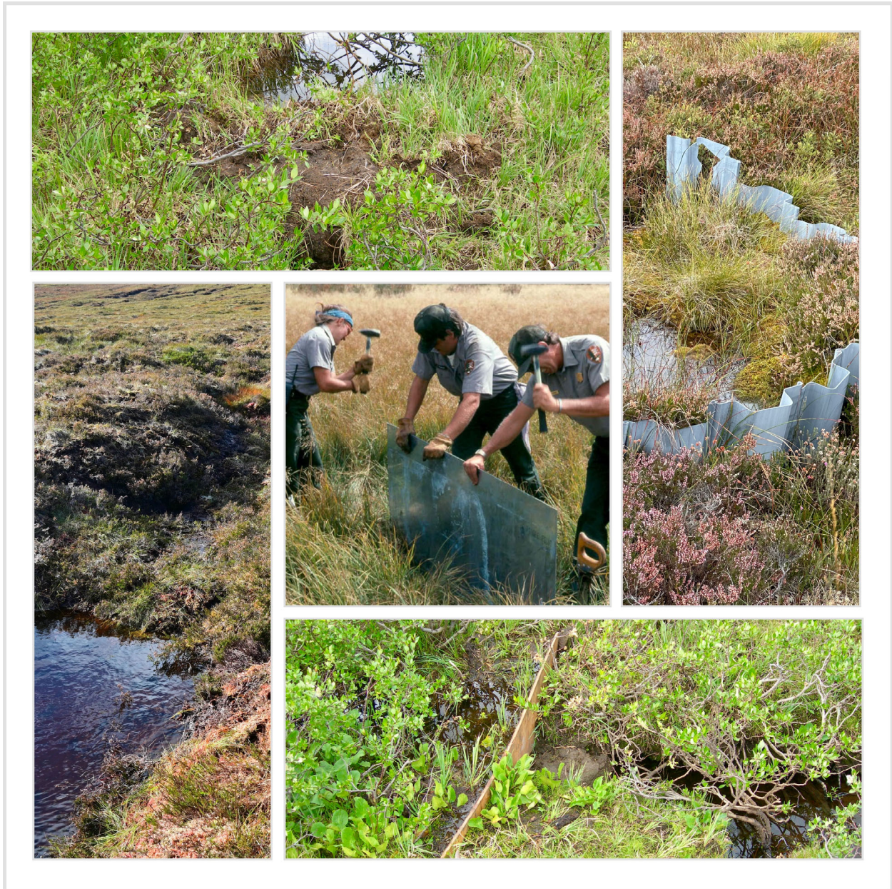
Figure 24. Examples of impermeable ditch dams to be used in low flow ditches. Peat dam (top left and bottom left), plastic (top right), steel (center), and wood (bottom right). Notice the degrading plastic (top right) from UV.
