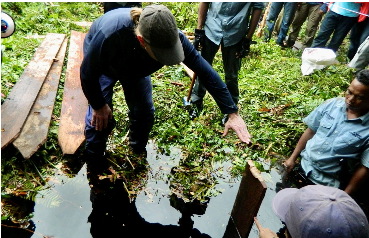
Figure 27. Vertical wood dams being installed in an Indonesian peatland. Notice the V-shape cut on bottom of the planks to facilitate pounding them into the peat. The first plank has been installed in the middle of the ditch with following planks installed adjacent to the first plank.
