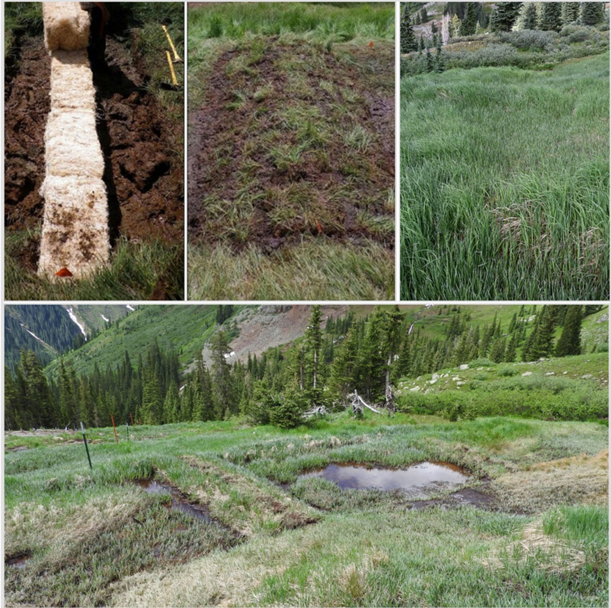
Figure 26. Example of how to build living ditch dams using bales for low flow ditches. A trench is dug and bales placed (top left) followed by peat sod being placed on the bales (middle right). After 1 year the sedges covered the bales and held it in place (bottom). Several years later, the dense sedge cover completely hid the bales (top right).
