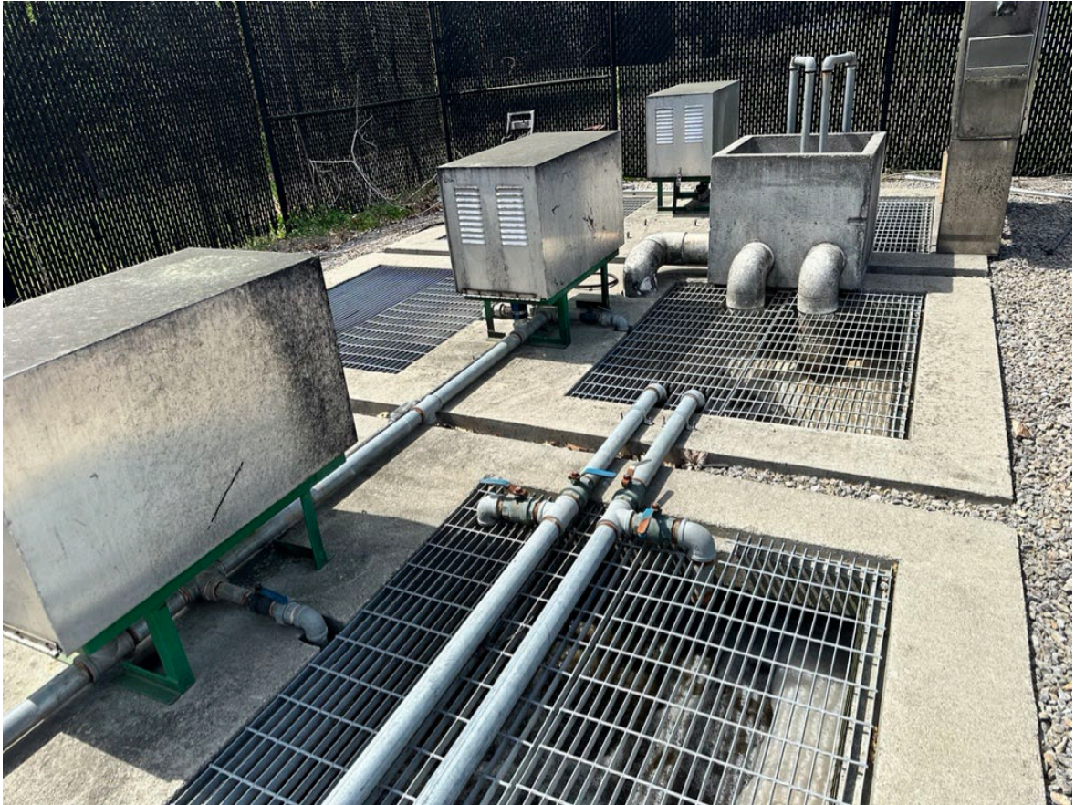
Figure B 1 Schematic of package wastewater treatment plant at the Central Kentucky Distillery's Bottling Facility.
