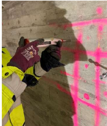
Figure 39: Schmidt-hammer test being carried out at one of the Kalix' bridge walls
