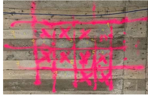
Figure 36: Layout of bars and tendons of one of the Kalix' bridge walls
