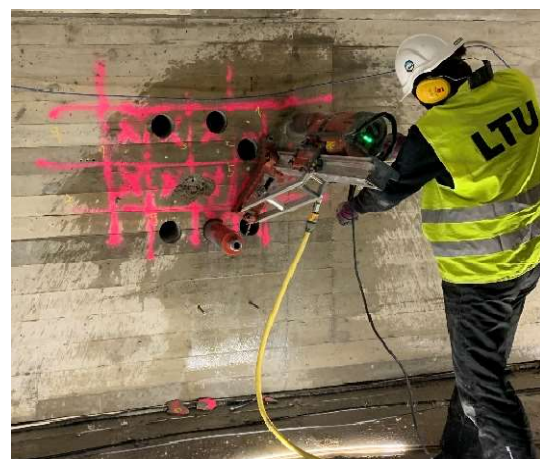
Figure 38: Core sample extraction process with the diamond coring tool for wet drilling (Hilti DD 200-CA Core Drill) at the Kalix bridge
