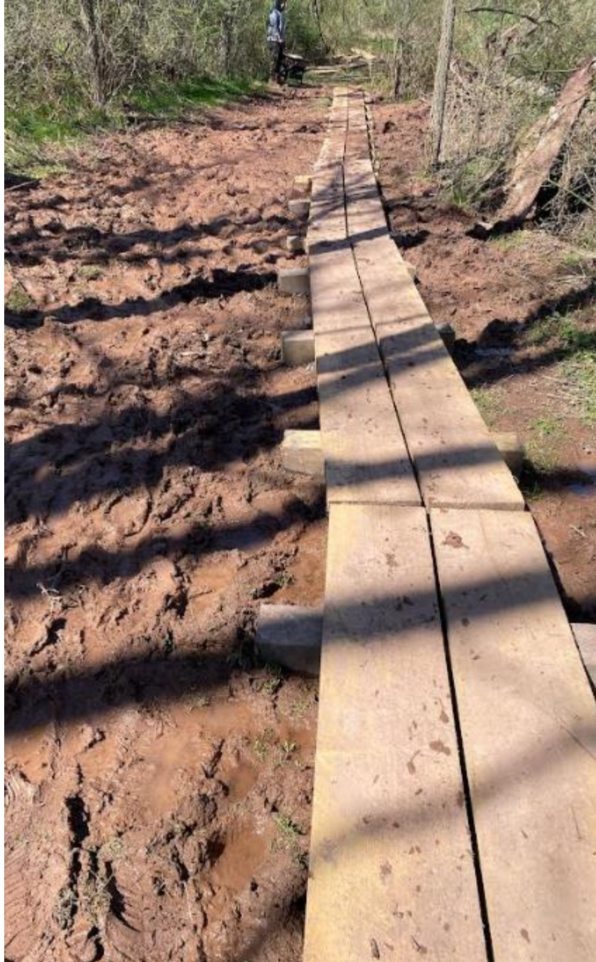
Figure 6. A picture of the puncheons constructed at Turtle Creek park based on the images and structural techniques provided to the team by Brian Aumann.
