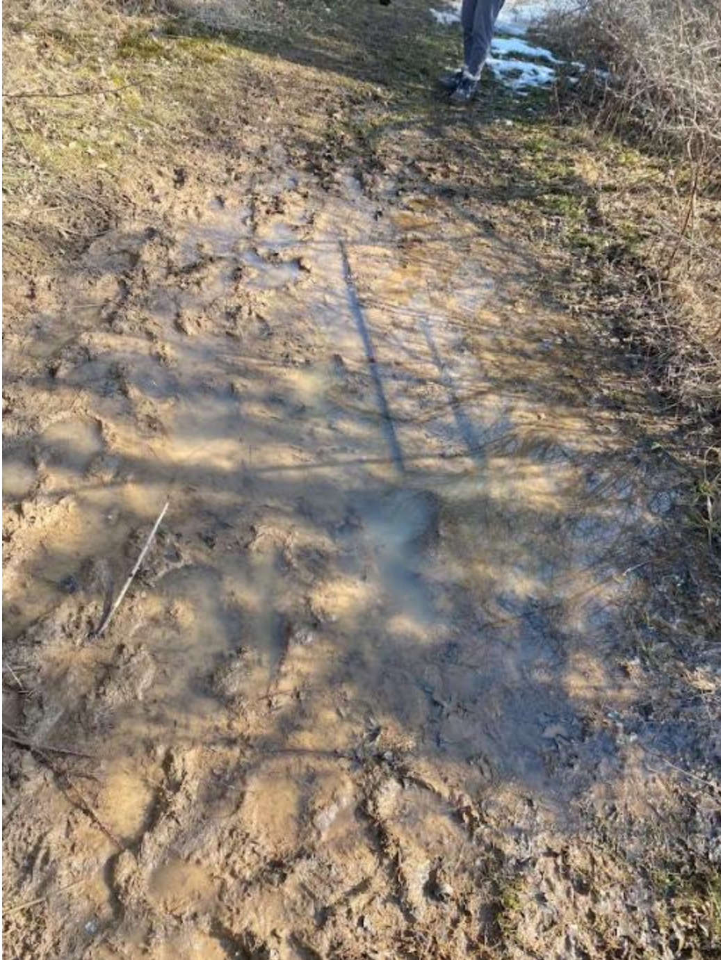
Figure 9. An image depicting an area along the north end of the Turtle Creek Park which is almost completely flooded and about 0.6 miles from the entrance of the park.
