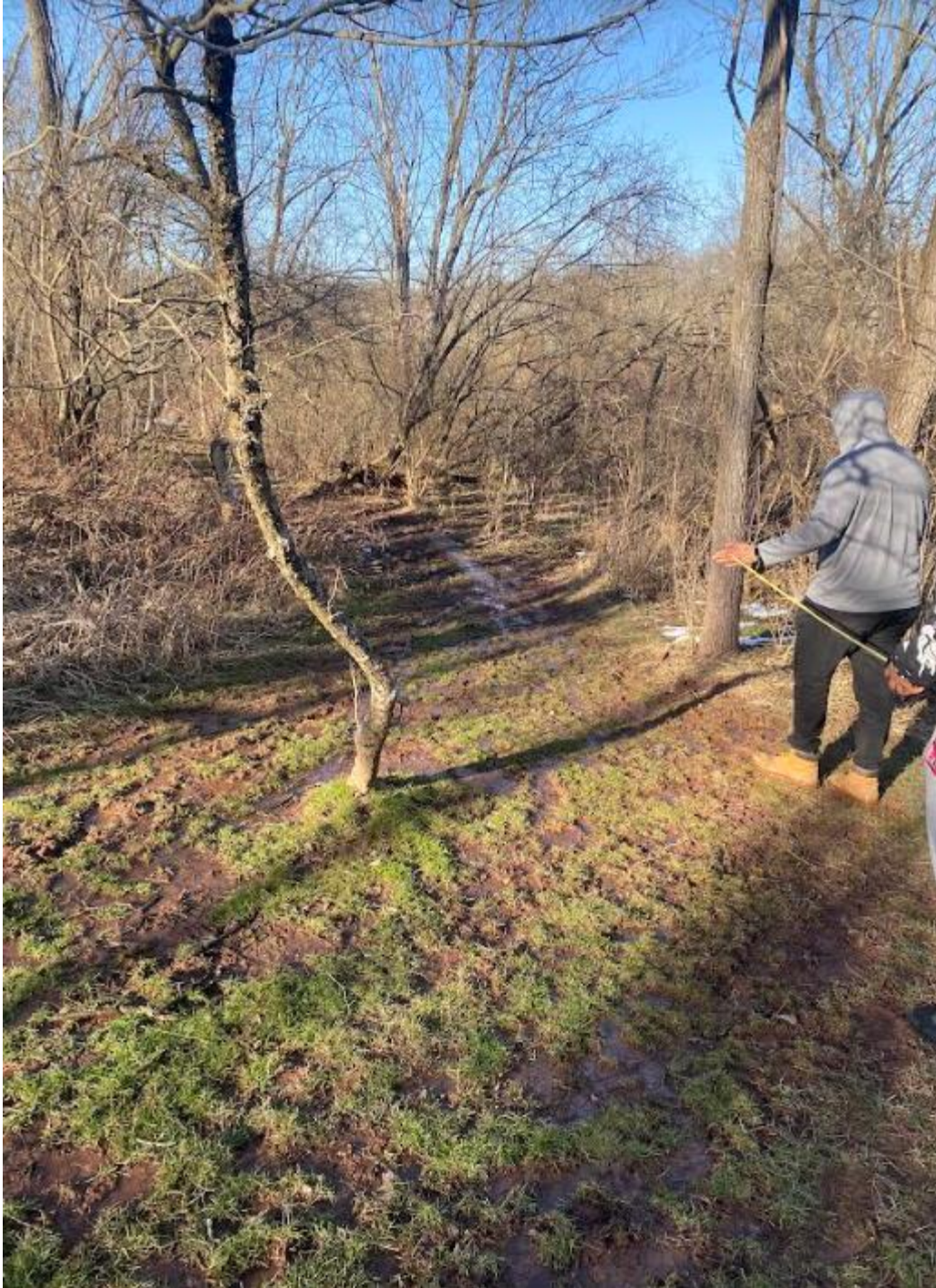
Figure 8. An image depicting the flooded conditions of one of the regions on the North end of the Turtle Creek, about 0.5 miles from the entrance of the park.
