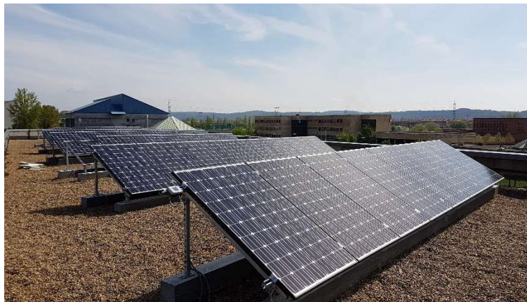
Figure 3.23. Main PV plant of the ERESMAGrid.
