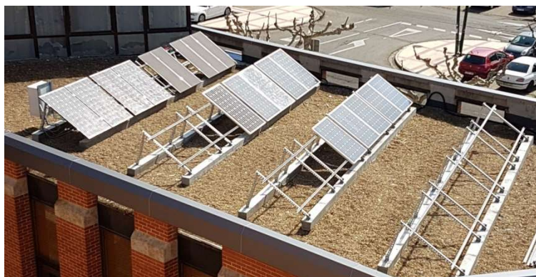
Figure 3.24. Test platform for PV technologies of the ERESMAGrid.
