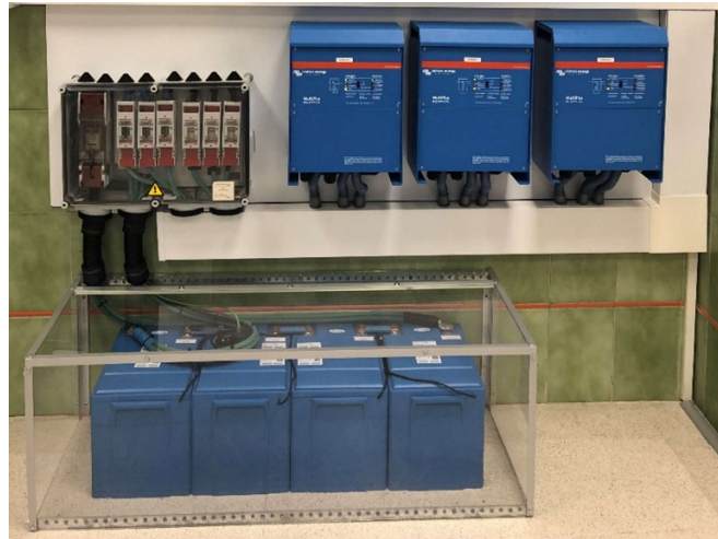
Figure 3.26. LiFePO 4 battery bank of the ERESMAGrid.
