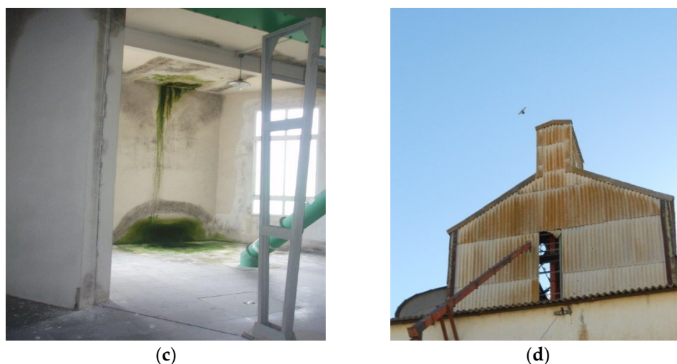
Figure 5. The state of conservation of the secondary network silos in Castilla y León is very diverse: the silos located at Tordesillas, Valladolid ( a ), and Alcañices, Zamora ( b ), are well preserved, whilst other silos present serious structural deterioration because of leaky roofs (silo at Nava del Rey, Valladolid: c ) or lack of vertical enclosure (silo at Piedrahita de Castro, Zamora: d ).
