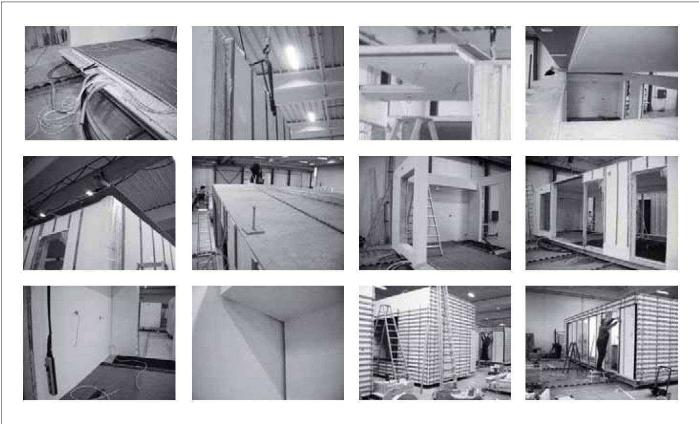
Production research at Boel Living, assembly of planar deck, wall and roof elements into complete volume-elements, fall 2007.
