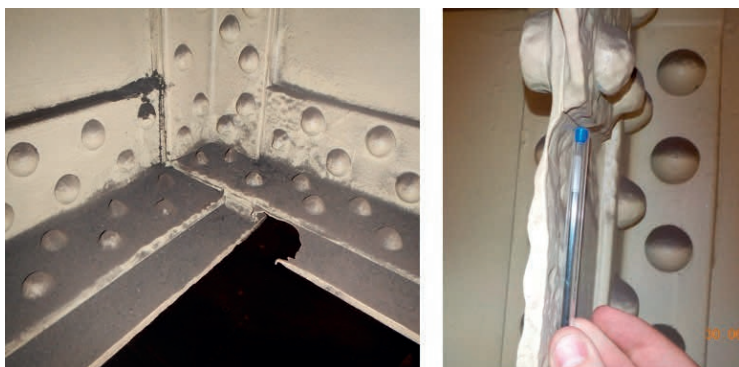
Figure 2.8: Localised corrosion (a) and heavy pitting (b) on the Boyne Viaduct
