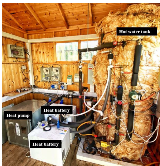
Fig. 15. Cascaded heat pump indoor unit with the commercial heat battery and the HWT thermal store test rig
