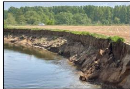
Active bank erosion showing erosion of sandy point bar deposits (June 2022)
