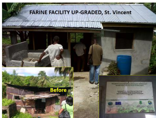
Figure 6. Refurbished farine processing facility in St. Vincent and the Grenadines
