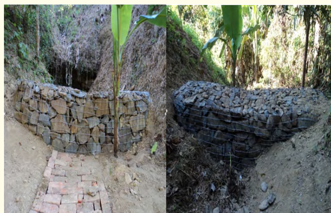
Figure 6: Gabion Check Dam (Front View at the left & Back View at right with Apron), Photo Credit: A. M. Zahid, SRDI.
