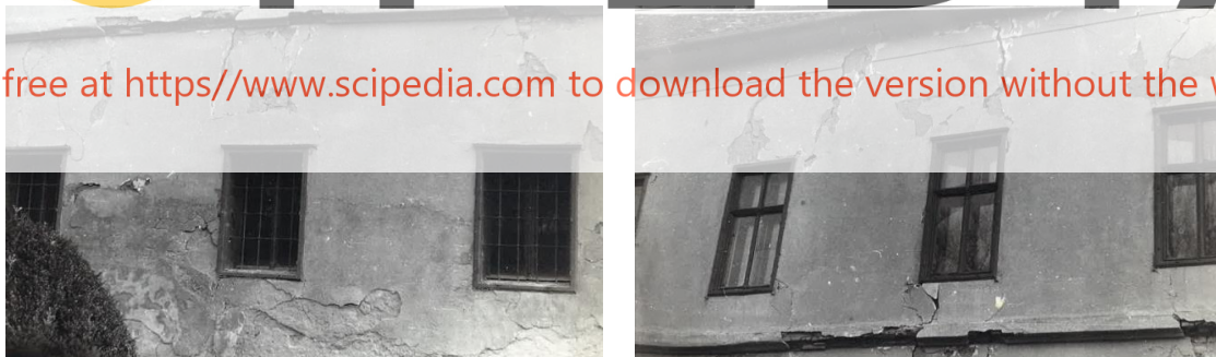
Figure 9: Vertical and diagonal shear cracks detected in the South façade of the case study building [19].
