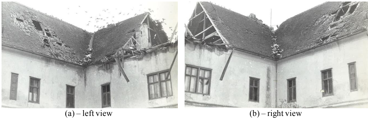
Figure 10: Failure mechanisms observed in the internal court of the case study building [19].
