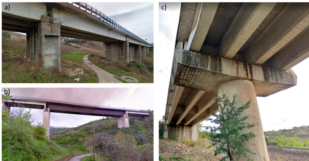
Figure 5. (a) Typical PRC viaduct, (b) steel span of a viaduct and (c) circular piers with cap beam.
