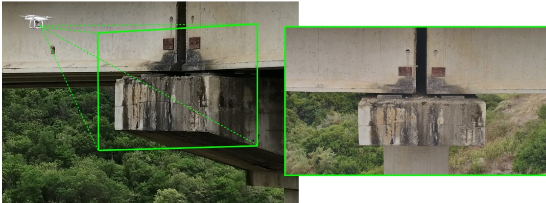
Figure 6. Visual inspection of the side of the structure by RPAS in manual mode.
