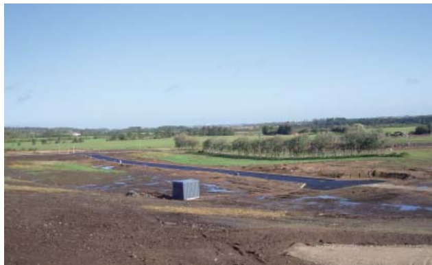
Figure 4.3.: Area for single family housing which has just been prepared (own photo).
