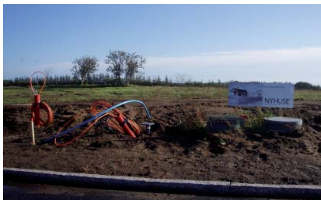
Figure 4.5.: The supply of electricity, water, sewage and phone for a lot for single family housing (own photo).
