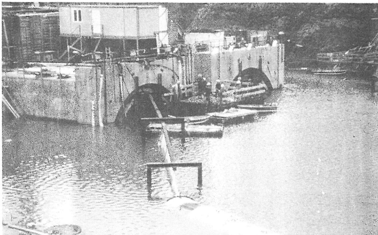
Fig. 23 Jutlandia incident with inundation of the tunnels and ramp on Sprogø 14 Oct. 1991
