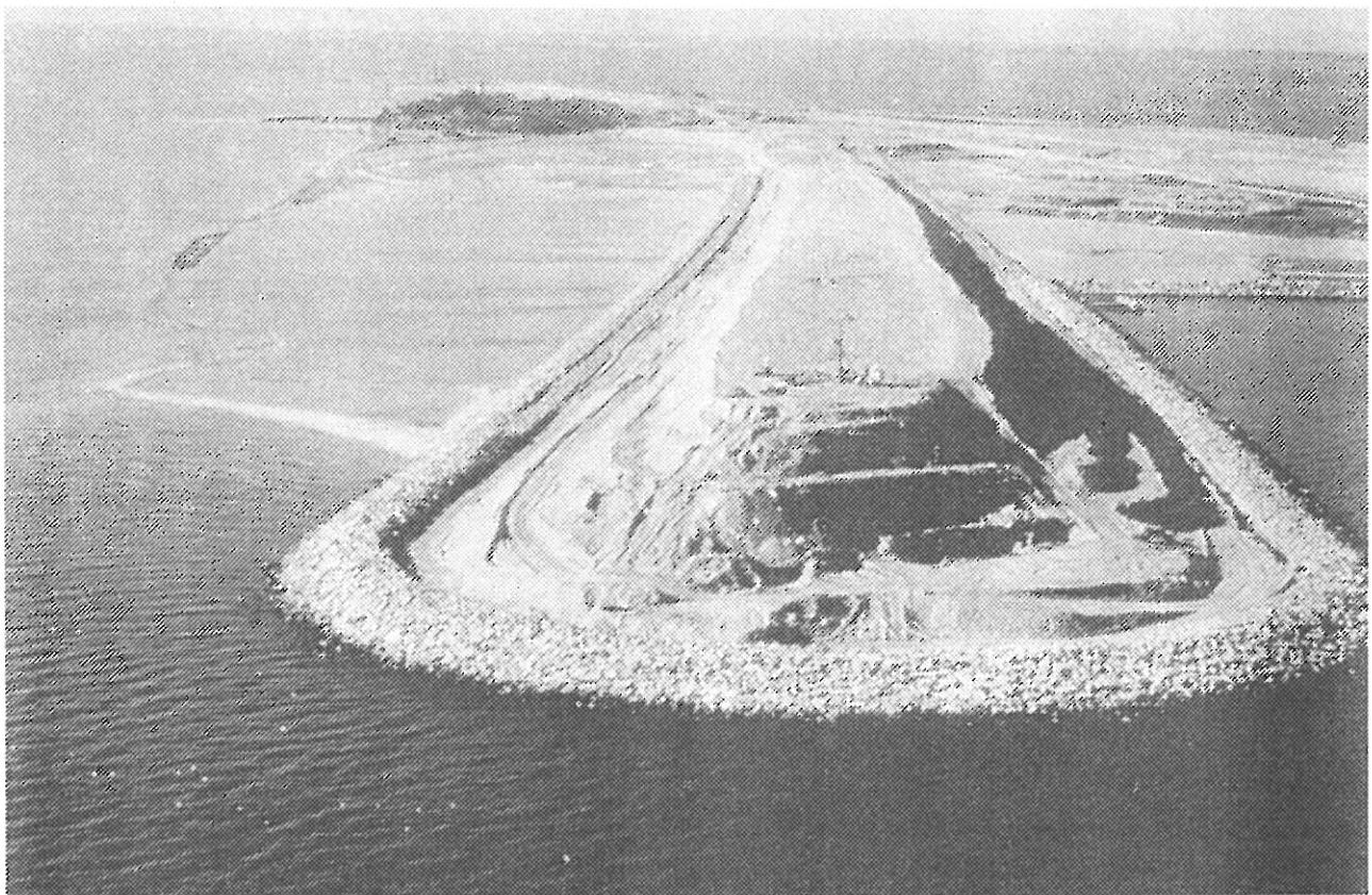
Fig. 22. DGI mobile drilling rig at top of embankment for East Bridge approach ramp on Sprogø
