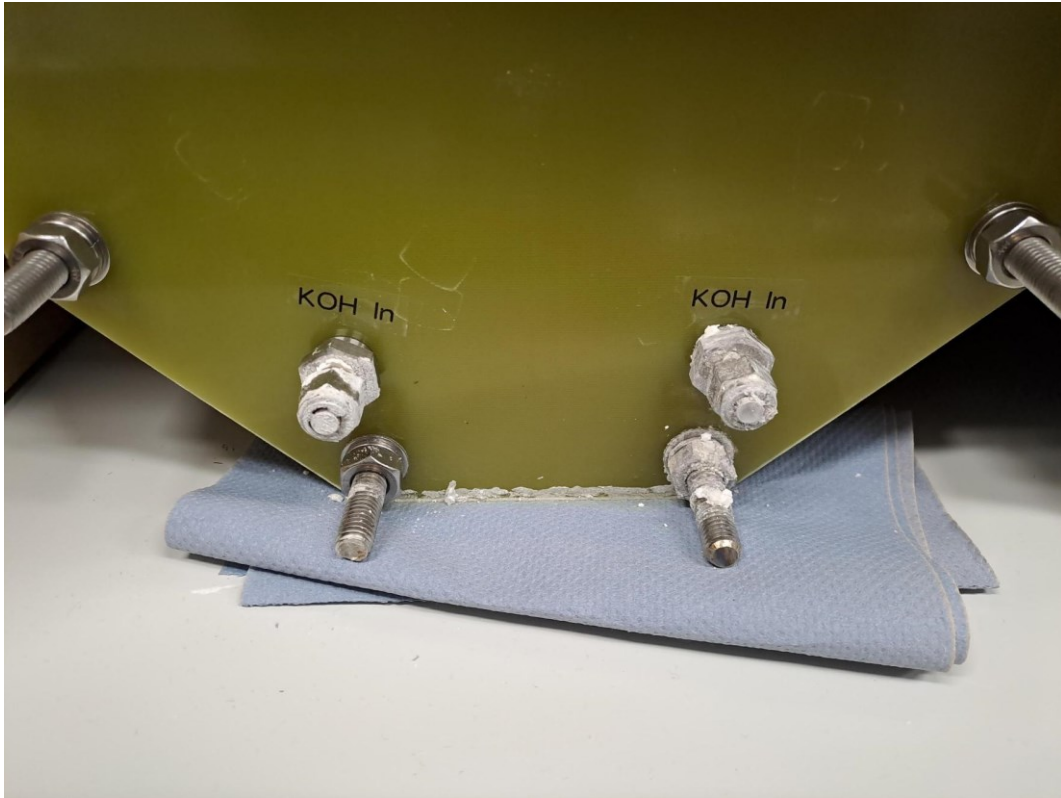
Figure 23. Solidified KOH on the stack inlets.
