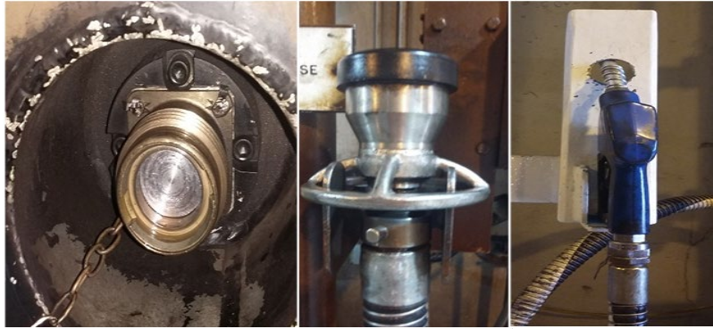
Figure 2.3 Various fluid ports and couplers used for train fluid servicing
