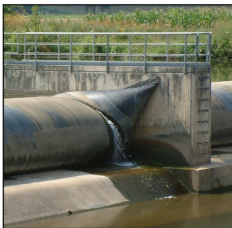
FIGURE 15 Rubber dam. Undesirable fold at abutment pier—major head water loss.
