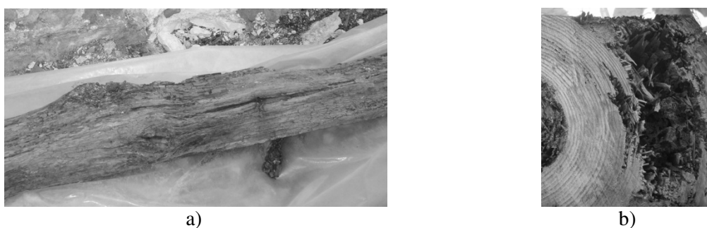
Figure 2.5: Example of a decayed timber element: a) along its length and b) a decayed cross-section
