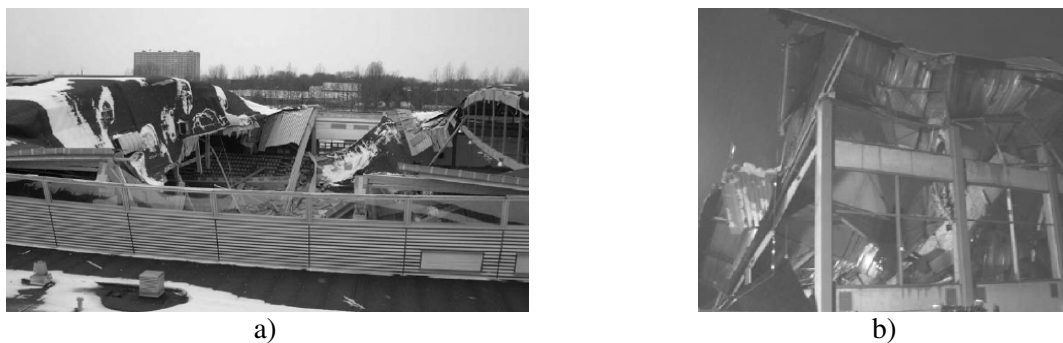
Figure 5.2: Structural collapses of glulam structures: a) Siemens Arena roof [Munch-Andersen e Dietsch, 2009]; b) Bad Reichenhall Ice-Arena, [Dietsch et al, 2009]
