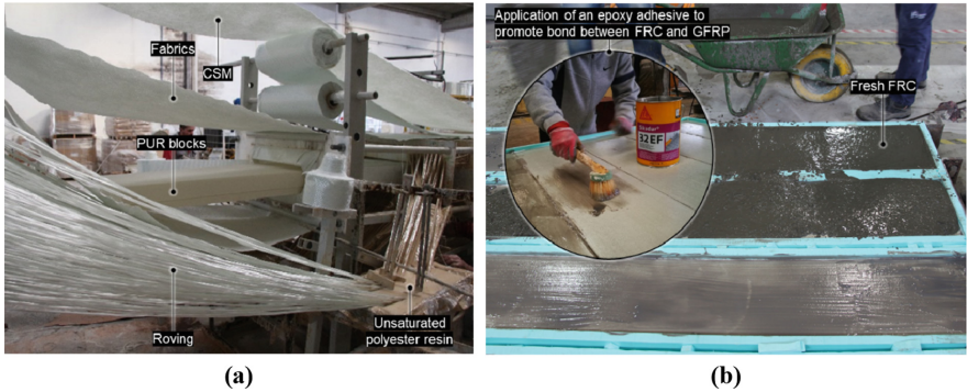
Fig. 4. Production of the sandwich panels: (a) pultrusion process and (b) FRC casting
