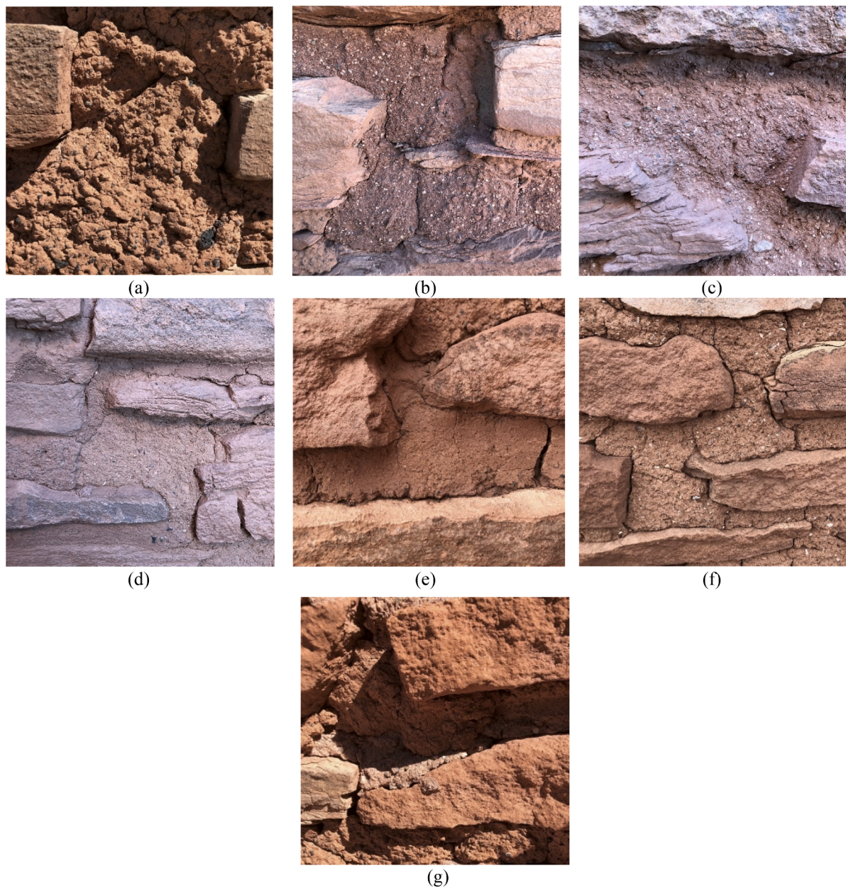
Fig. 9. Types of mortar identified on-site: (a) EM1; (b) EM2; (c) EM3; (d) EM4; (e) EM5; (f) EM6; (g) CM.
