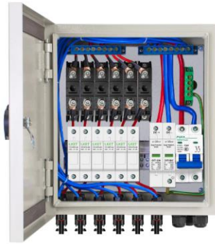
Figure 25 – Example of a string combiner box.
