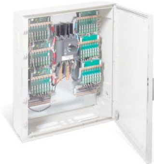
Figure 110 – Example of a string box (Schneider Electric, 2016).
