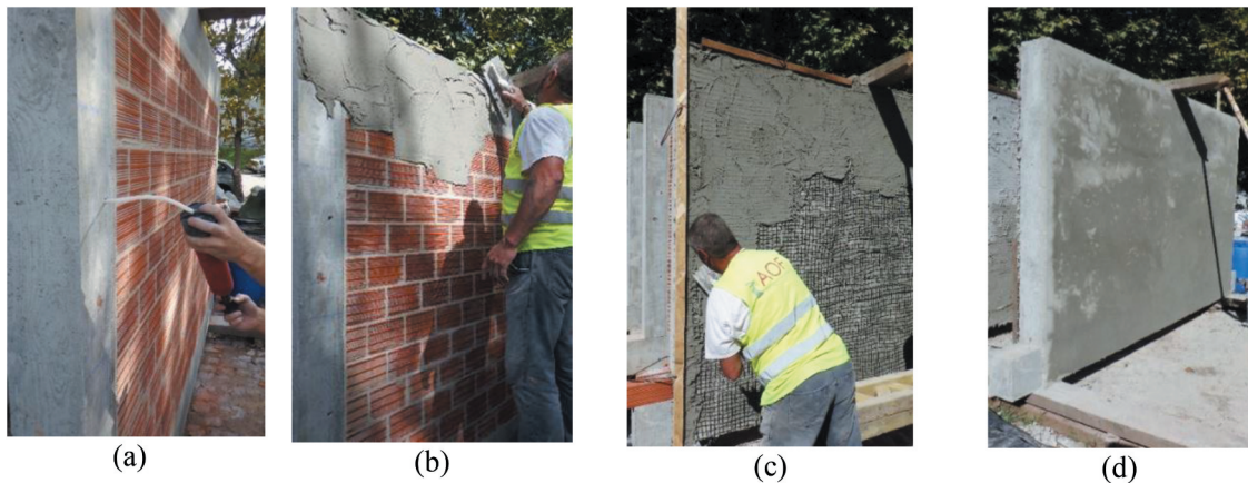
Figure 5. Application of the reinforced rendering; (a) drilling the pilot holes, (b) applying the first layer of mortar, (c) positioning of the textile mesh and application of the second layer of mortar, (d) final aspect after rendering.
