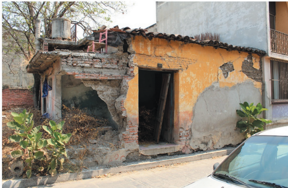
Grade 3: Substantial to heavy damage (moderate structural damage, heavy non-structural damage).
