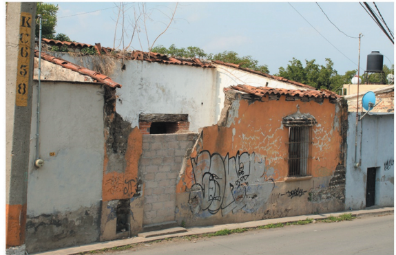
Grade 4: Very heavy damage (heavy structural damage, very heavy non-structural damage).
