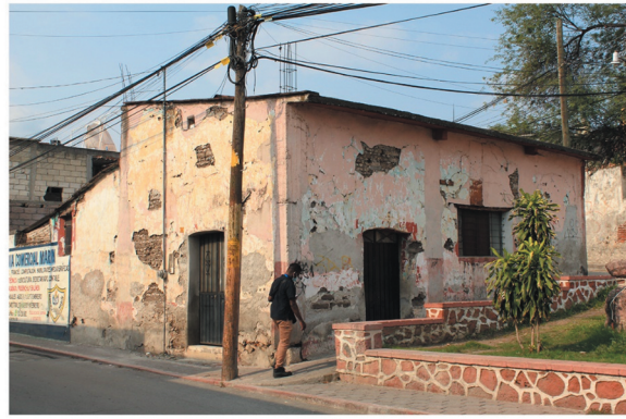
Grade 2: Moderate damage (slight structural damage, moderate non-structural damage).
