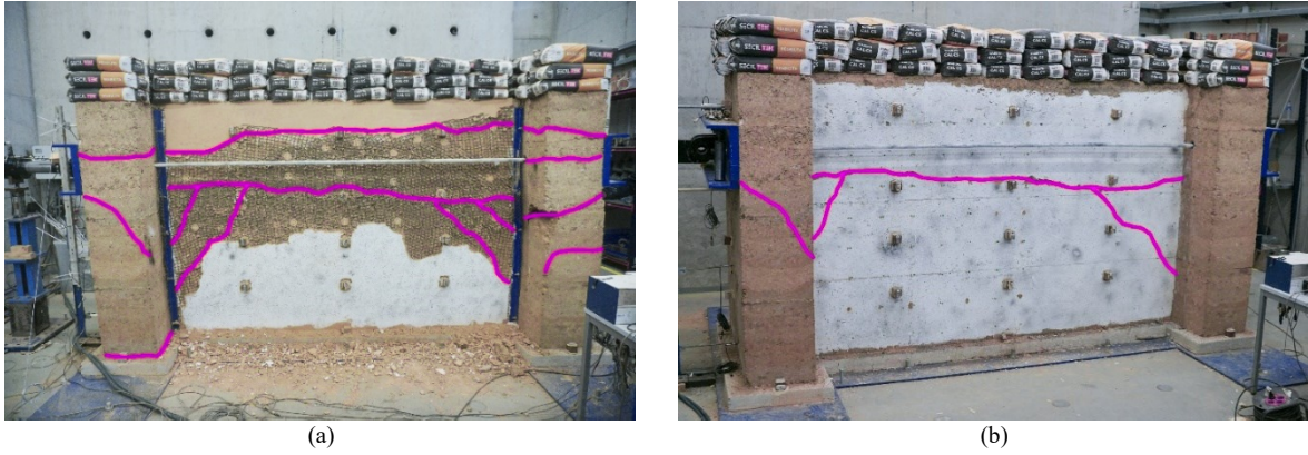
(a) (b) Fig. 9 Cracking pattern of: a) GeoRE-IP model, and b) URE-IP model.
