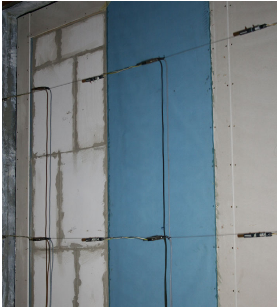
Figure A12. After mounting a vapour barrier on the indoor side of Element 3. At the left Element 4 (cellular concrete), at the right Element 2 where no vapour barrier was mounted. Suspended RH sensors (Rotronic) are seen in front of the elements.
