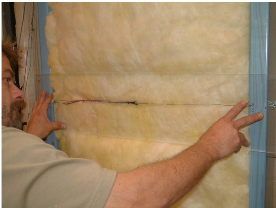
Figure 7. Placement of moisture sensors in fixed positions in the insulation layer.
