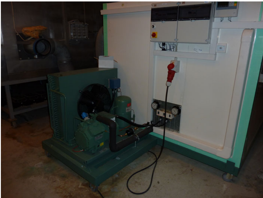
Figure A19. Cooling machine and compressor.
