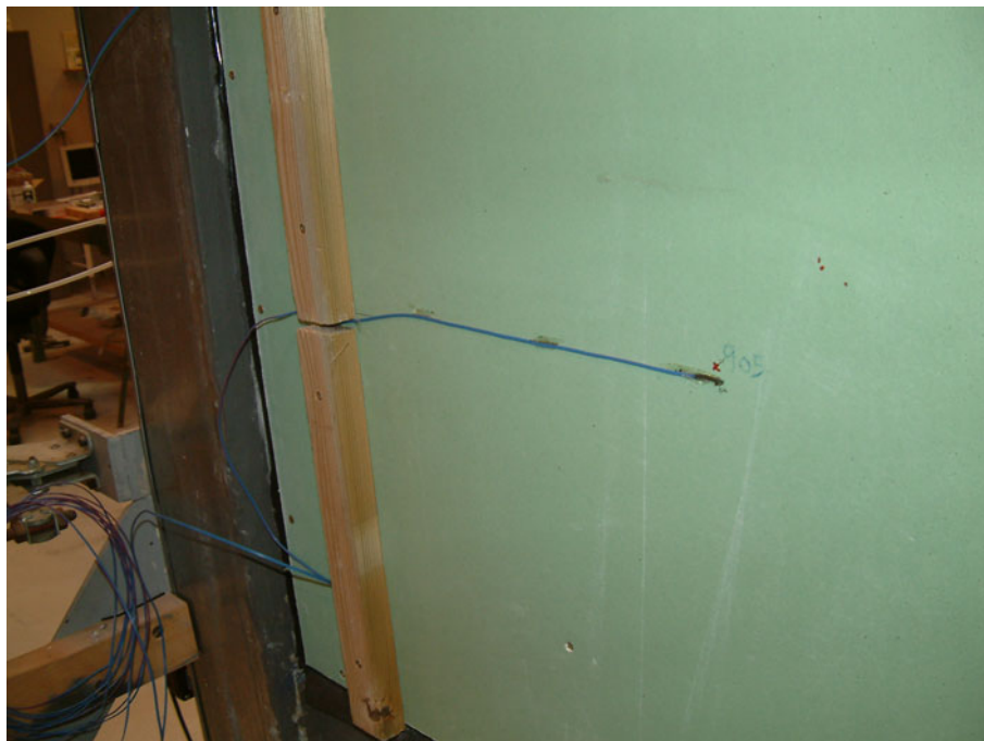
Figure 8. Fixing of sensors at the outdoor side of the wind barrier.
