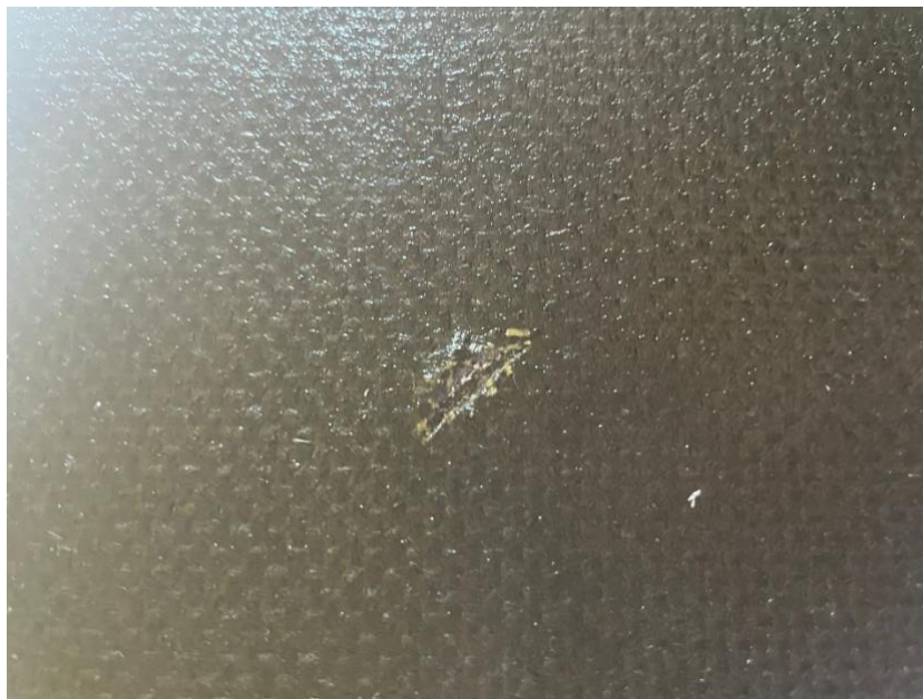
Figure 1. The general appearance of the damage
