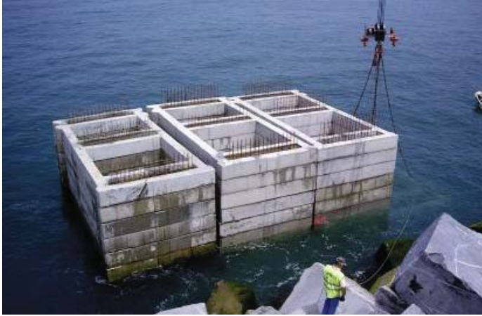
Figure 13. Installation of the OWC caissons composed by 16 pre-fabricate slides, Mutriku, 6 m water depth.
