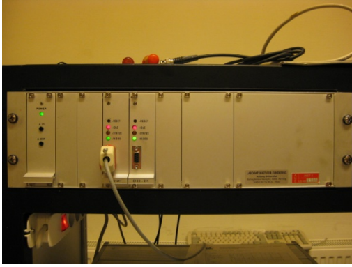
Figure 3.2 Front side of PSC-rack.
