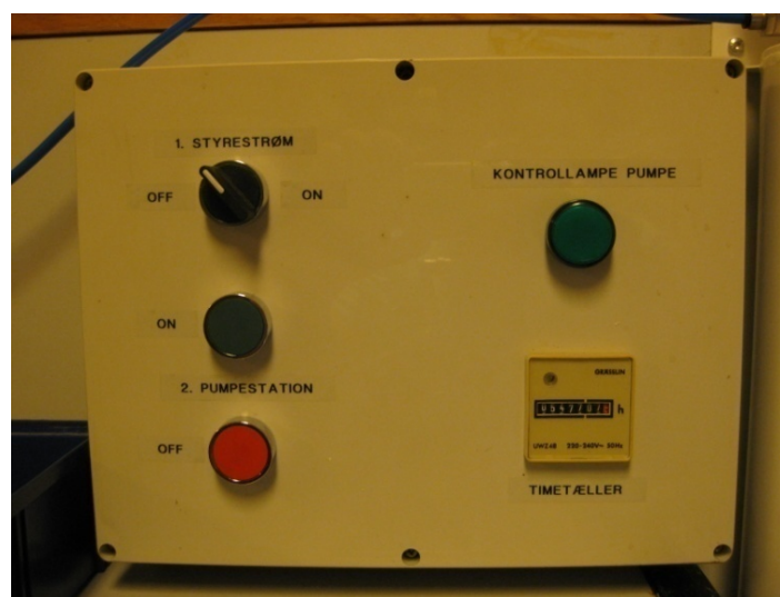
Figure 2.3 Circuit breaker panel for hydraulic pump.
