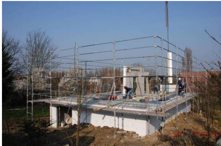
Figure 18: Installation of peripheral scaffoldings before the installation of the walls. (Foto: Frédéric Bougrain).
