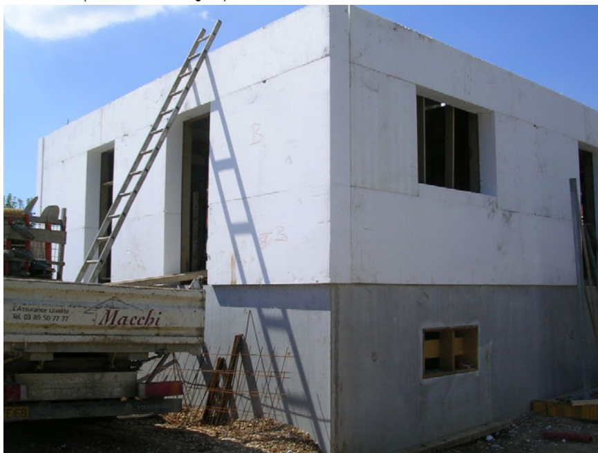
Figure 19: With prefabrication there is no more waiting period for interior paintings or the roughcast of the facades. (Foto: Frédéric Bougrain).
