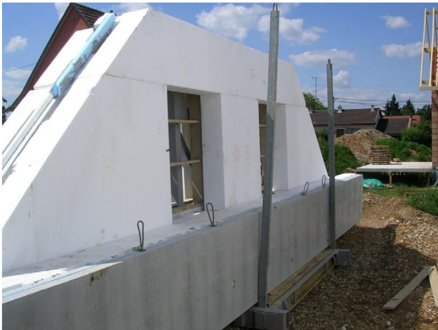
Figure 16: Prefabrication and strong external insulation allows to achieve better energy performance. (Foto: Frédéric Bougrain)
