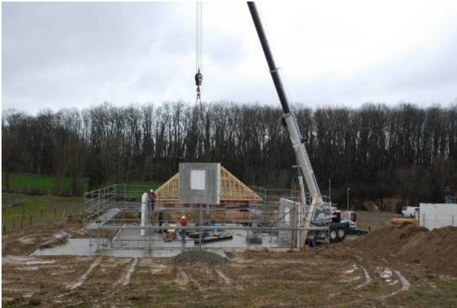
Figure 20: The use of cranes of strong tonnage to install prefabricated walls improves working conditions and reduces on-site risks. (Foto: Frédéric Bougrain).
