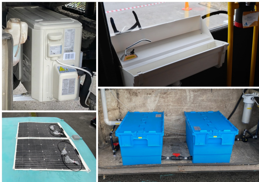
FIGURE 5 Clockwise from left: Roof-mounted modular solar panel system, retrofitted air-conditioning unit, indoor low-profile sink with a water dispenser and rainwater collection tanks with a water filtration system.
