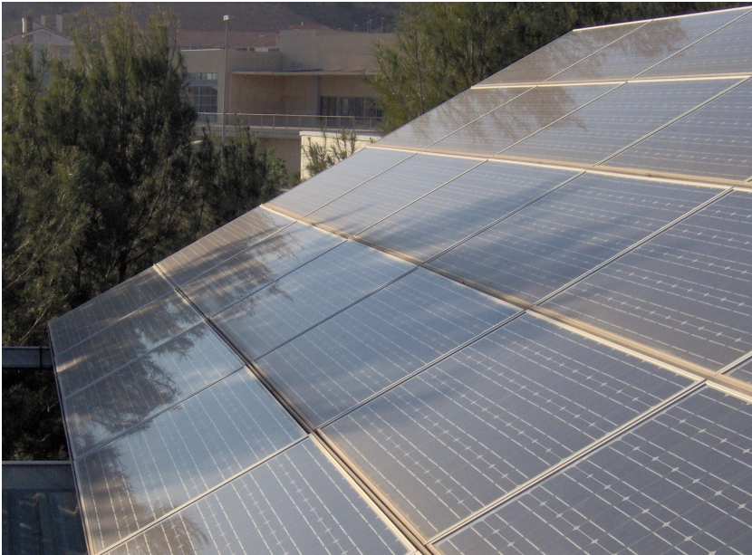
FIGURE 1.8 CRYSTALLINE SILICON MODULES INSTALLED AT UNIVERSITY OF MURCIA
