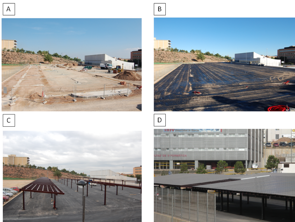
FIGURE 4.7. BUILDING PROCESS OF 222kWp CDTE PARKING FACILITIES: (A) EARTHWORKS, (B) MASTIC ASPHALT, (C) METALIC STRUCTURE ASSEMBLY AND (D) STRUCTURE-INTEGRATED CDTE MODULES PLACEMENT AND FINAL WIRING AND GRID CONNECTION. THE SYSTEM ALSO INCLUDES INFORMATIVE PANNELS ABOUT THE FACILITY FOR TEACHING PURPOSES.
