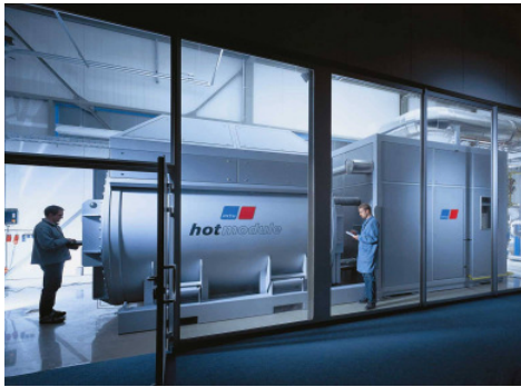
Installation at a Hospital at Bad Berka, Germany
