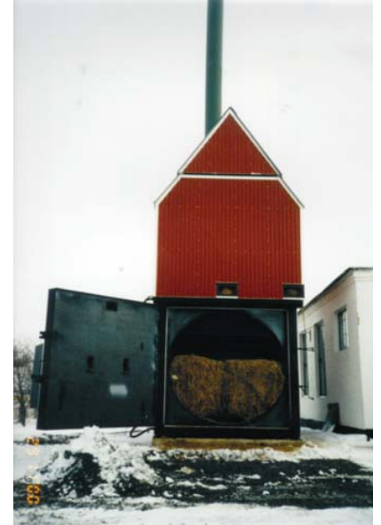
Fig. 3: 980 kW straw fired boiler in Kyiv oblast. Design of PASSAT, Denmark.
