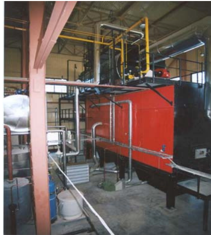
Fig. 2: 5 MW wood fired boiler at veneer plant Odek-Ukraine. Design of KARA, the Netherlands.
