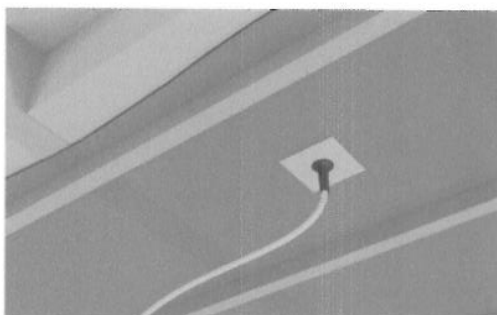
Figure 6. Ceiling-mounted conduit for wiring. The airtight shell of the entire ceiling was attached to the conduit. The airtight shell in the ceiling was established by a polyethylene foil that also served as a vapour barrier. The polyethylene foil was placed between the wood trusses and the laths. The frame of the conduit was joined to the polyethylene foil.
