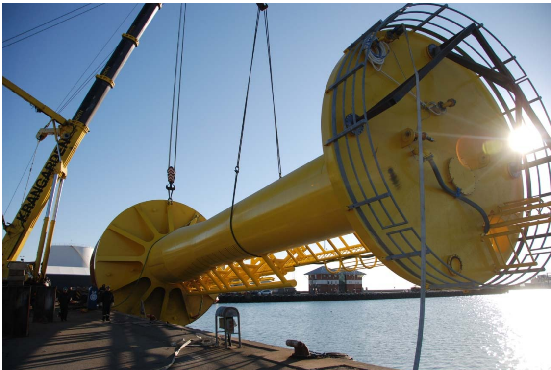
The first monopod bucket foundation, the Mobile Met Mast, to be installed offshore, Denmark, 2009
