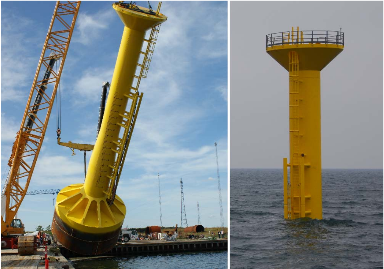
Fig. 18. Successful installation of the Mobile Met Mast at Horns Rev 2 Offshore Wind Farm, Denmark in 2009.
