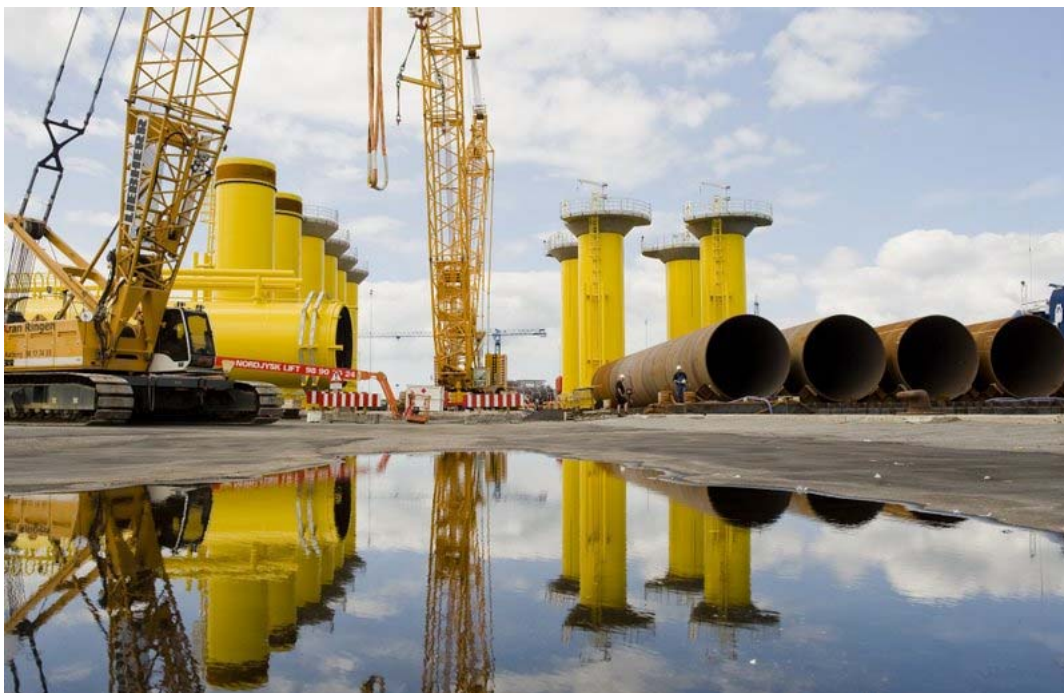
Fig. 5. Construction yard for fabrication of monopiles for Horns Rev 2 Offshore Wind Farm, Denmark, 2008.
