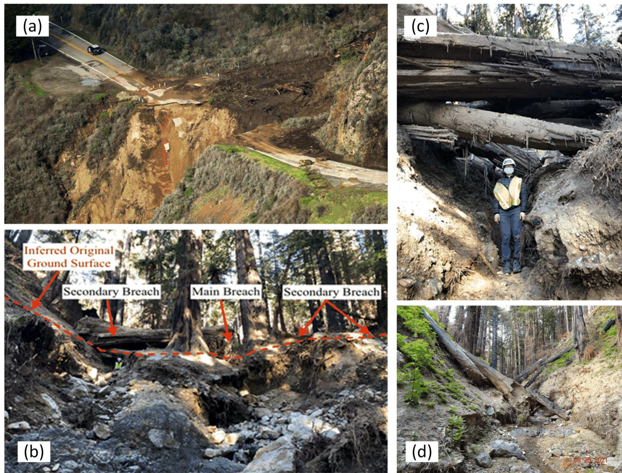
Figure 3. Highway one Embankment Failure Following the Dolan Fire, CA. (a) Aerial photograph showing a V-shaped canyon created by the erosion of the Highway one embankment material, (b) Photograph showing the main breach area and secondary breach areas that likely occurred before the main breach based on observed scour and water retention, (c) Photograph showing one of the investigators standing at the entry point to the left secondary breach area and fallen tree trunks above for comparison purposes, and (d) View looking upslope within Rat Creek showing the eroded channel and residual burned tree trunks in and on the slopes of the creek.
