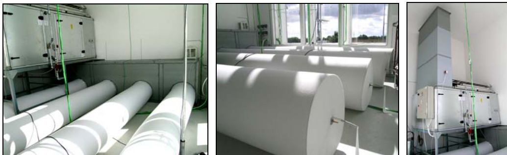
Figure 3. KE-low impulse fabric ducts in the experiment room (left, centre), Ventilation system in the experiment room (right).
