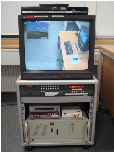
Rack in observation room.
