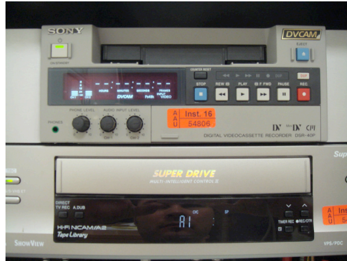
DV and VHS machines in the rack
