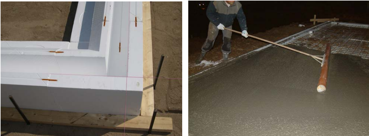
Figure 6 a): Left, prefabricated lightweight elements, made of EPS, mounted as the strip foundation. The elements were fixed together with large clamps of plastic, b): Right, 300 mm EPS, mounted as two layers on top of the base of stamped gravel bordered by the strip foundation that served as the insulation layer underneath the concrete floor slab. Iron was mounted as a net inside the strip foundation and as wires along the moat formed by the two vertical boards of EPS in the prefabricated elements, before concrete was cast and leveled.
