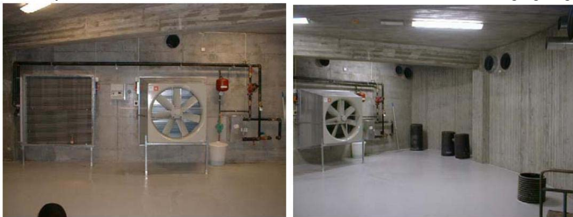
Figure 4.13. The air distribution room, showing the preheat unit (left) and fan, as well as the plastic subterranean ducts leading to the various rooms (Schild 2002a).
