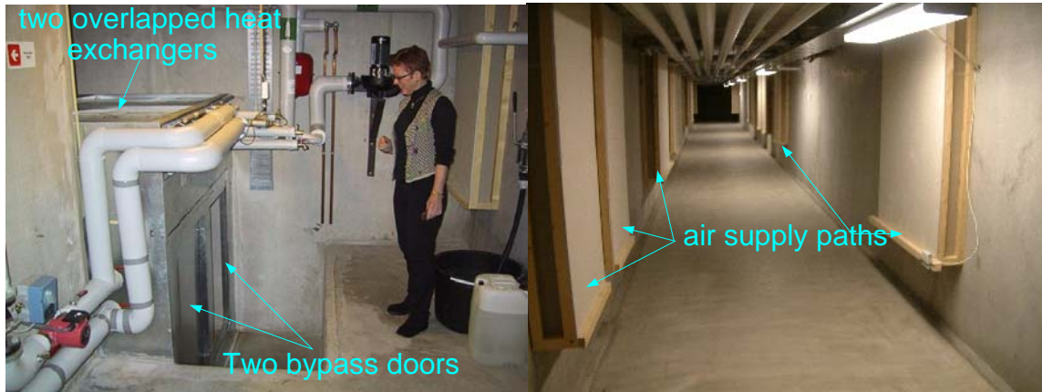
Figure 4.9. Air distribution duct of Mediå school (Left photo shows heat exchangers and “summer” doors. Right photo shows the supply air paths) (Tjelflaat 2002a).
