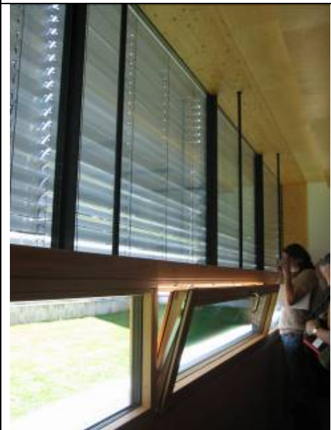
Picture of the façade in the classrooms. The external shading is automated, the automation can, however, be overruled by the users. Inlet openings are placed in the bottom in order to allow shading and ventilation simultaneously. The classrooms are also mechanically ventilated through inlet and outlet openings in the ceiling.
