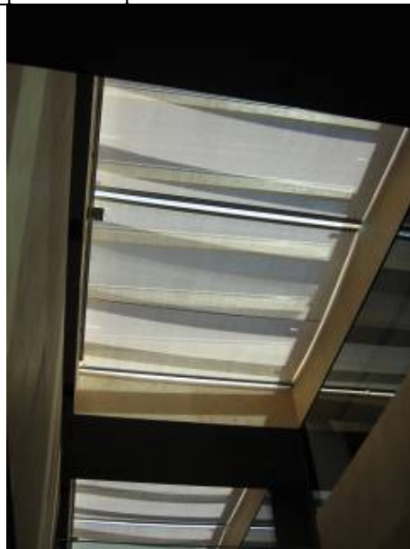
This picture shows the internal shading device in the atrium. The shading is activated when the temperature in the cavity is 40°C.
