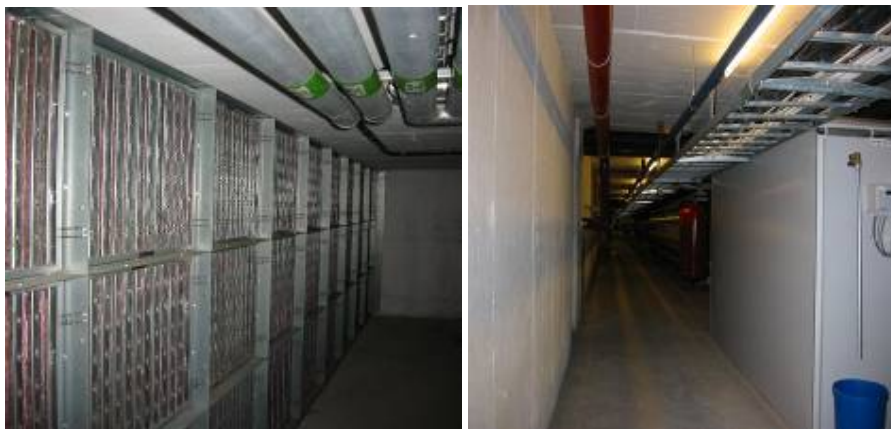
Filter at air intake in culvert (left) – low pressure drop. Storage tank for solar DHW is place in culvert (right). The culvert surfaces are painted.
