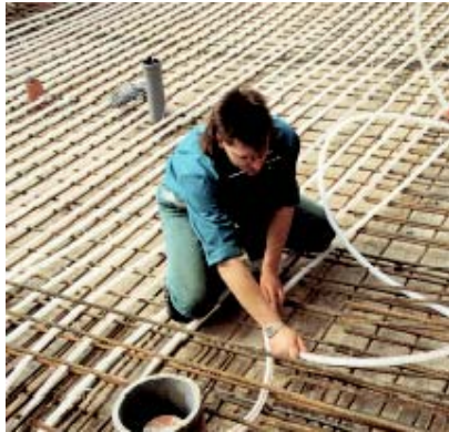
Installation of the pipes on the reinforcement grid of the future concrete floor slab (Hauser 2002)
