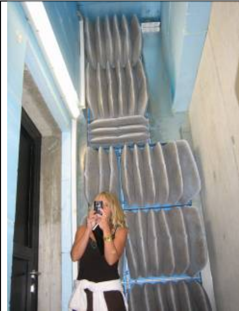
Picture taken of the inlet opening to the earth cooling.
