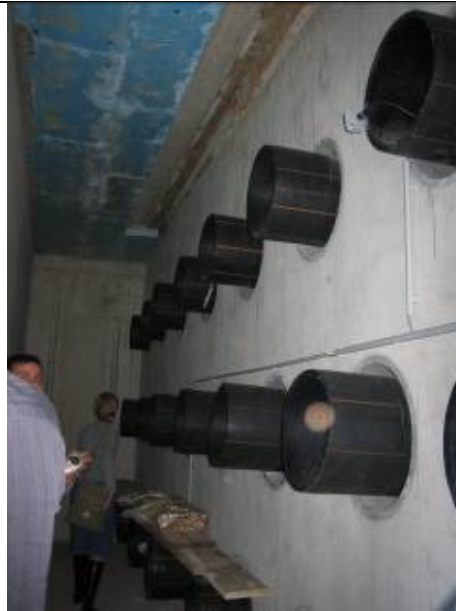
The picture shows the ducts through which the air is let into the basement area where the air is preheated or precooled.
