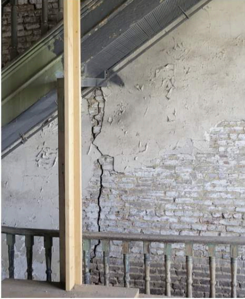
Figure 4.2 - Interior photo of structural damage due to foundation instability
