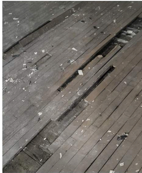
Figure 4.5 - Dilapidated wood flooring
