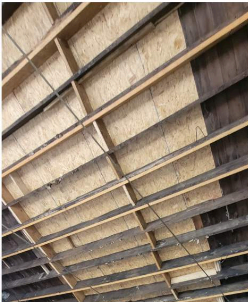
Figure 4.4 - Floor repair due to water damage
