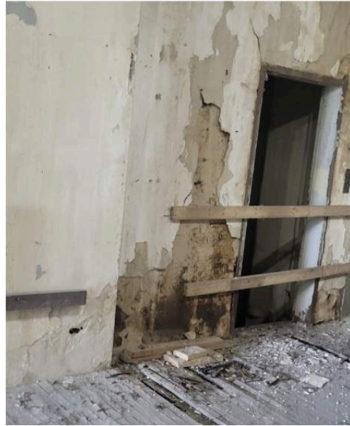
Figure 4.3 - Wall decay due to water damage
