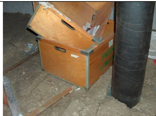
Dis-placed and compressed roof insulation.
