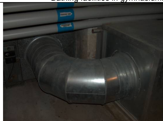
New, un-insulated ventilation system.
