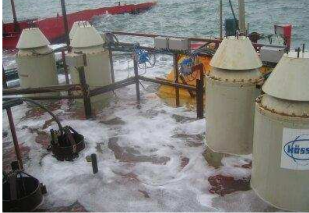
Fig. 11: Turbines in the reservoir of the prototype: The yellow structure in the background is the siphon turbine, the grey towers are five of the six cylinder gate turbines, and the small devices in unpainted steel are two of the dummy turbines.
