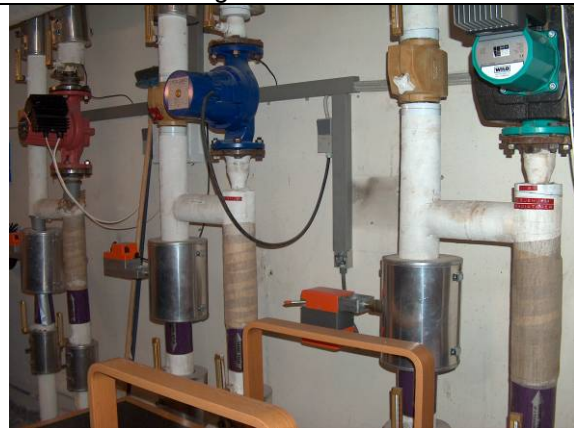
Heating distribution central.
