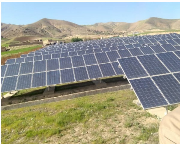
Figure 3. Solar Panels of Yeka Tut Village of Chal District
