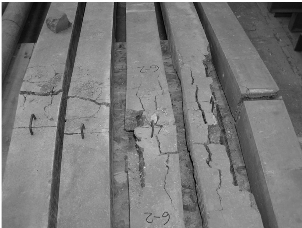
Figure 7 - Other columns tested at DTU. The one on the far right shows failure at a stirrup, while the centre column shows a cover to the reinforcement considerably larger than the nominal cover of 15 mm.
