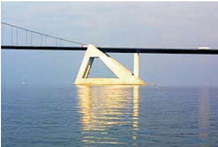
Figure 1.1 An example of a modern large geotechnical structure. One of the anchor blocks of the Great Belt Bridge. ( www.storebaelt.dk )
